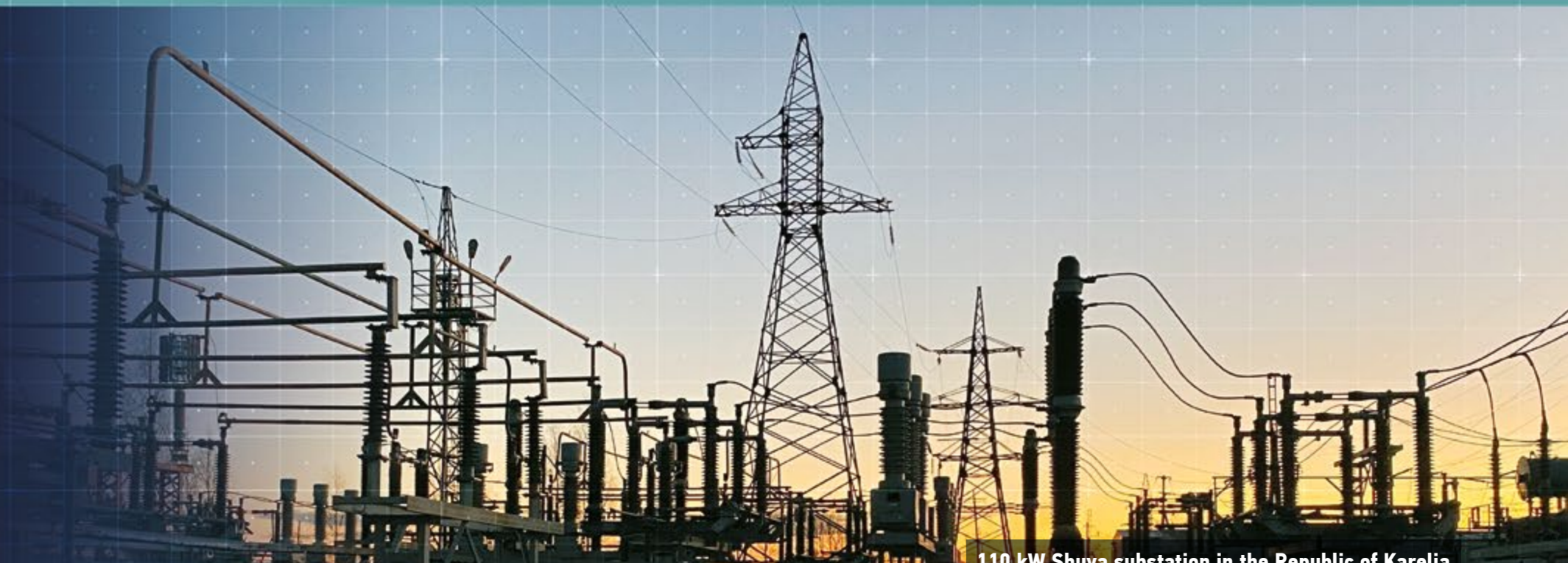
110 kV Shuya substation in the Republic of Karelia
